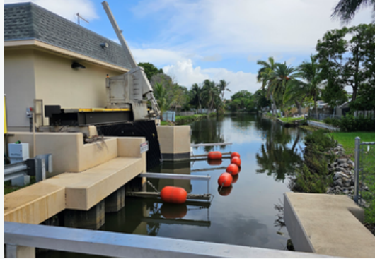
Storm Water Pump Station 3 which was heavily used during the week of June 10 floods in Hallandale Beach, FL (Photo courtesy of Mike Sukop).
